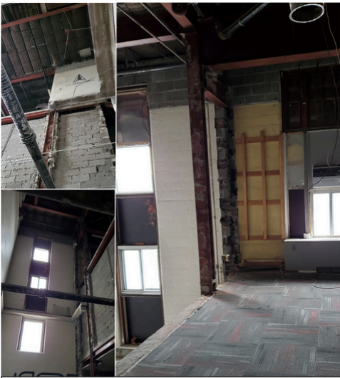
Commander's Office (right) to open stairwell on east side (left) for elevator
